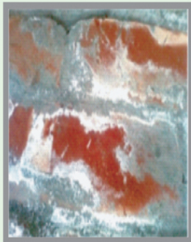
Salt on bricks surface
